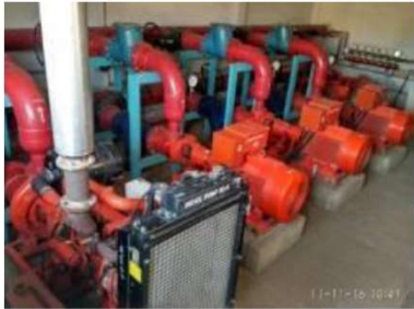
Fire Hydrant Pumps
