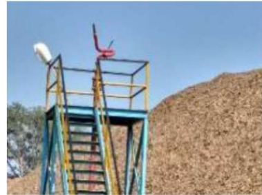
Fire Hydrant Point near chipper
