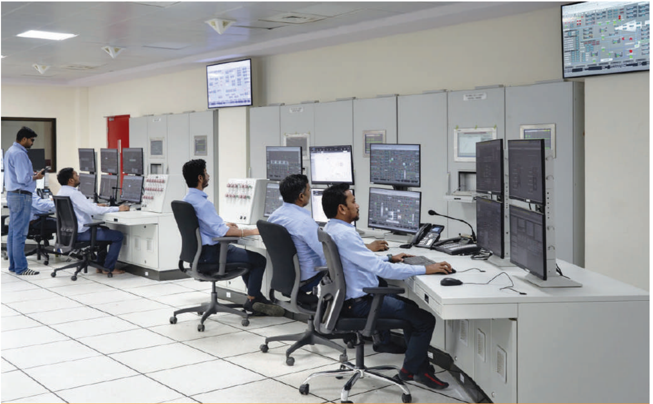
Main Control Room at Ammonia Plant, Talaja
