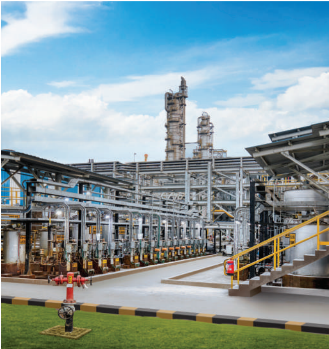
Reverse Osmosis (RO) Plant
