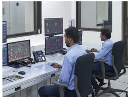
Water Control Room
