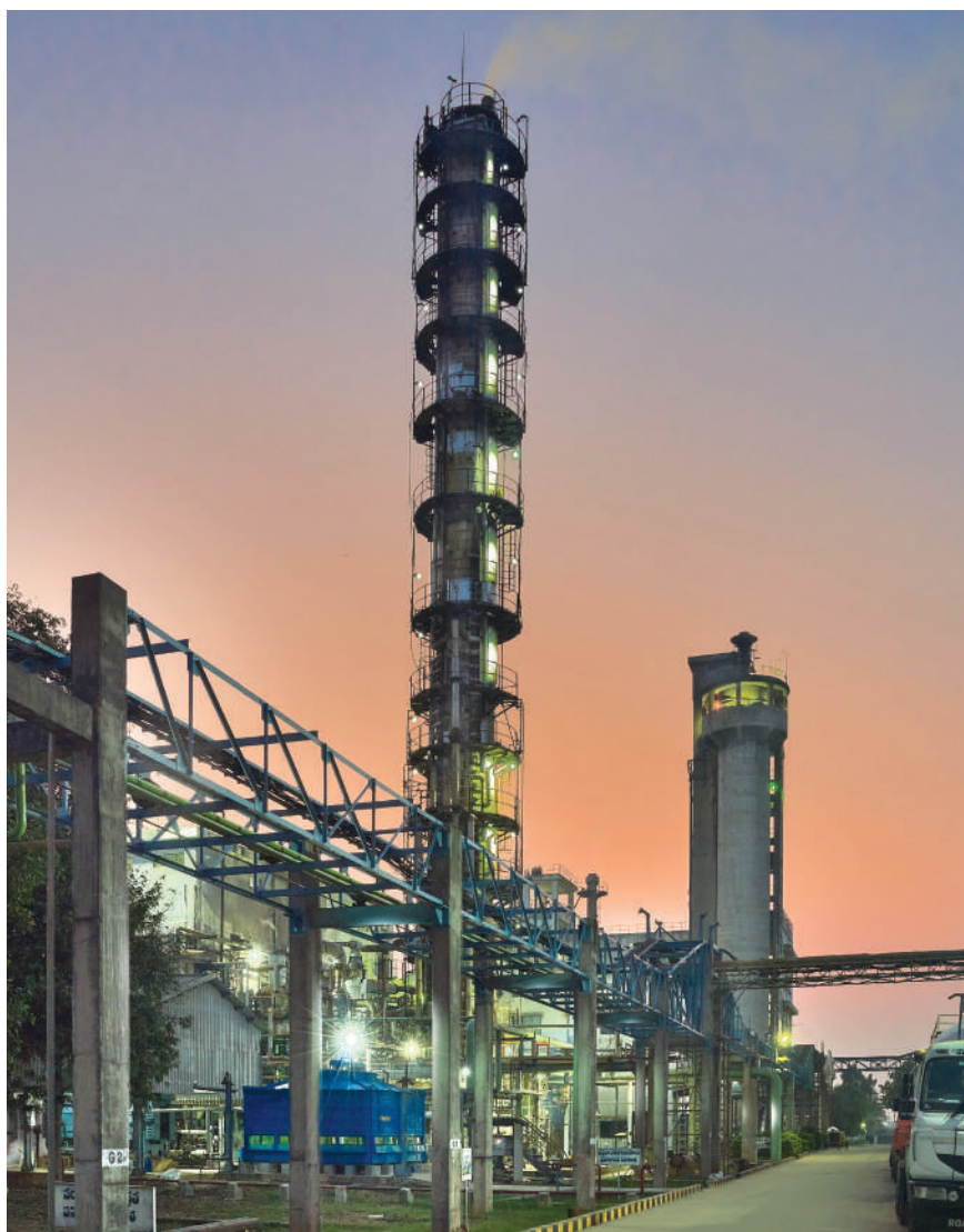
State-of-the-art Technical Ammonium Nitrate Plant at Srikakulam
