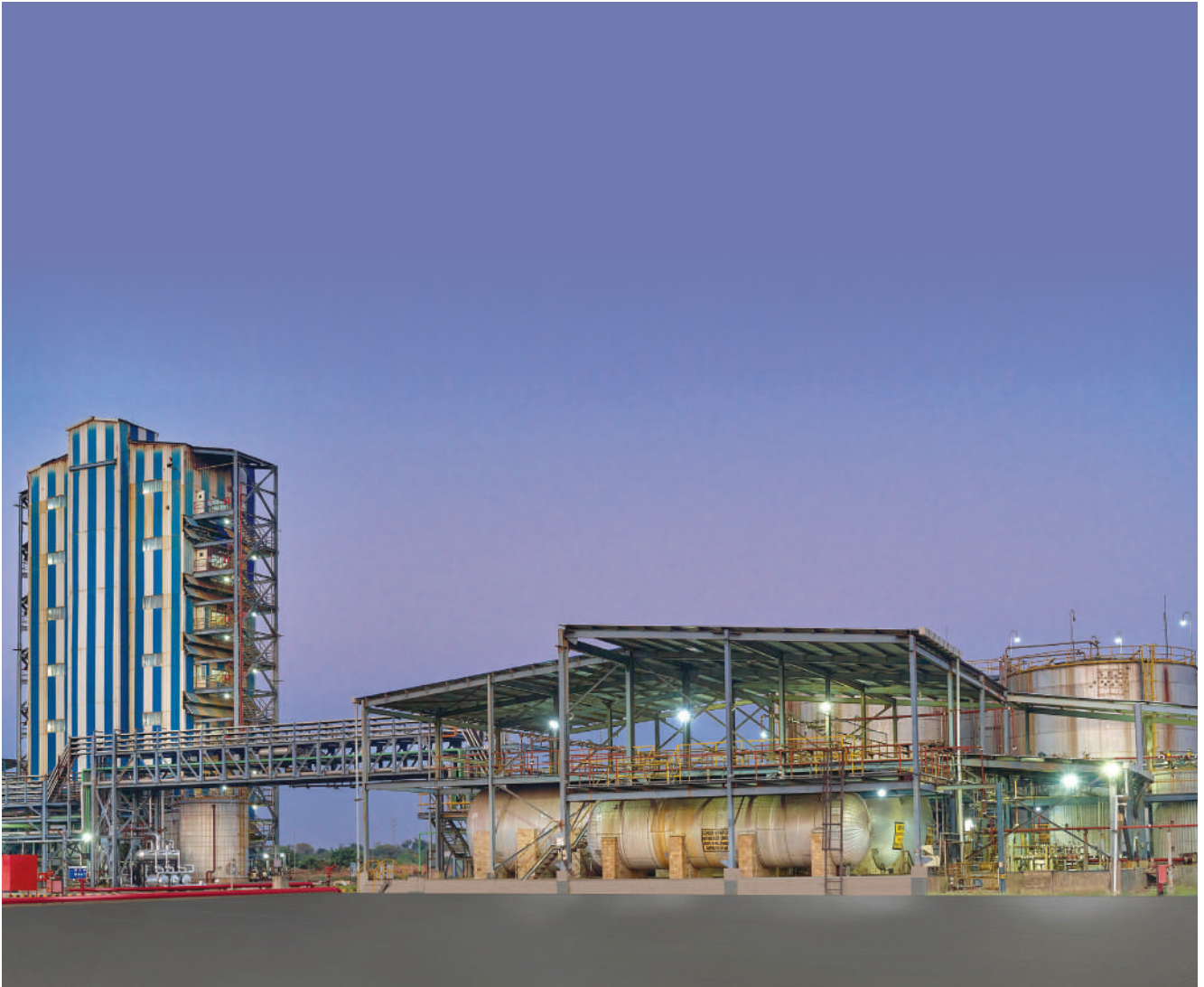
Concentrated Nitric Acid Plant and Storage Tank at Dahej
