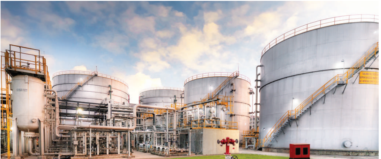
DM Plant and Water Storage Tanks
