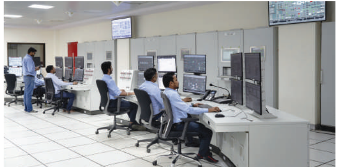
Main Control Room
