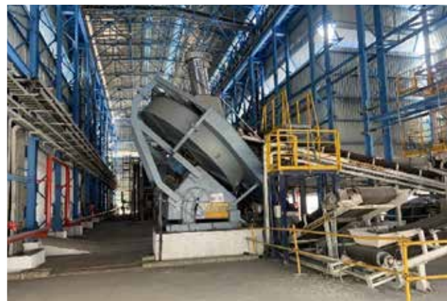
LWA Plant at NTPC Sipat
