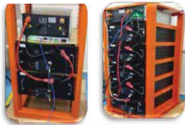
Energy Storage System (ESS)
