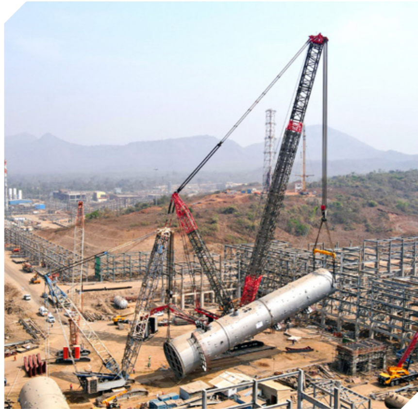
▶ SANY SCC16000A 1600MT crawler crane and Demag CC 2800-1 600MT support crane doing Splitter column section erection at Usar, Maharashtra site.
