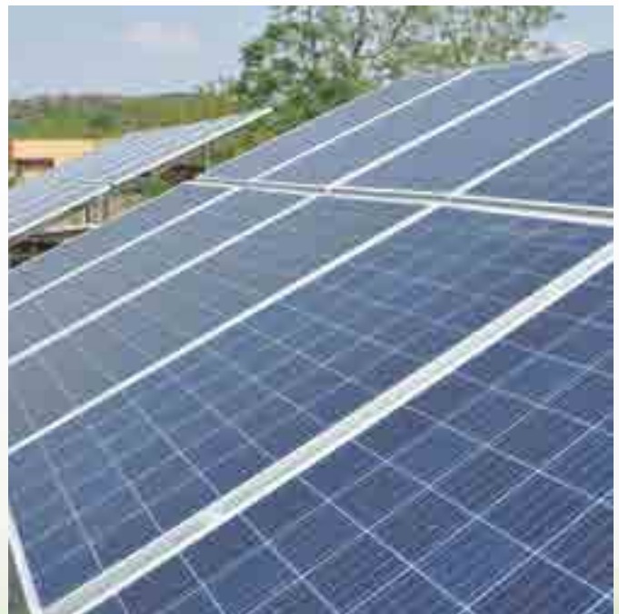
Solar panels in KCC
