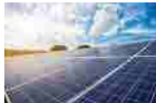
Copper in Solar plants
