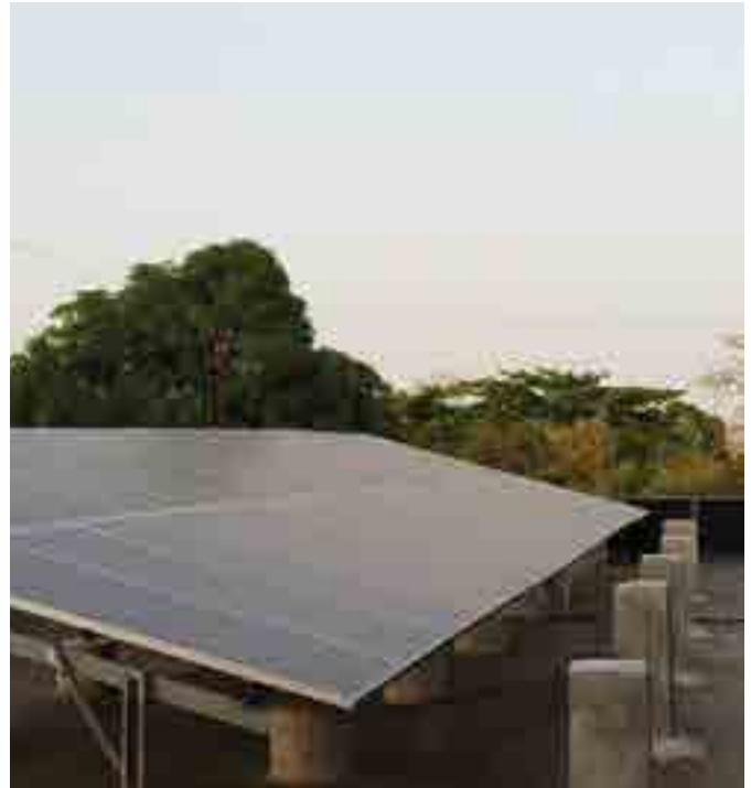
Rooftop solar plant in MCP
