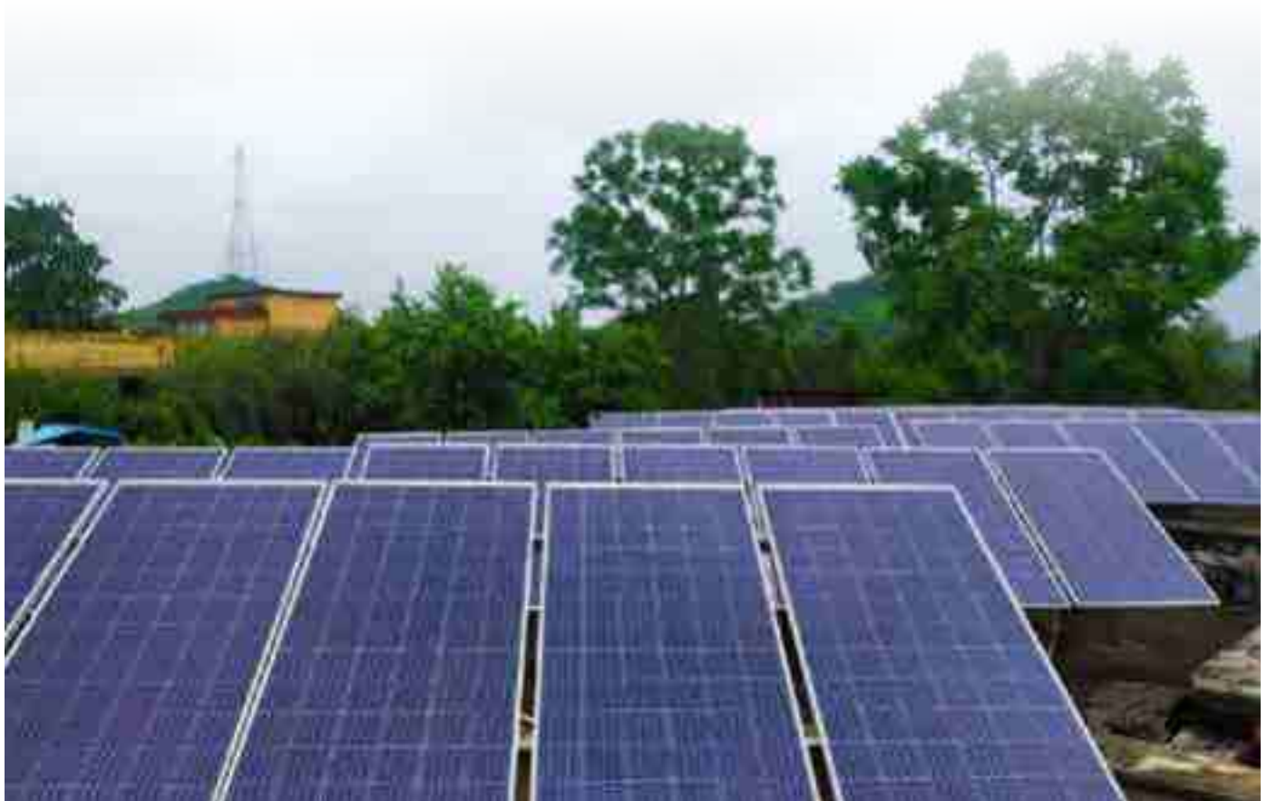
Solar panels installed at KCC Hospital.
