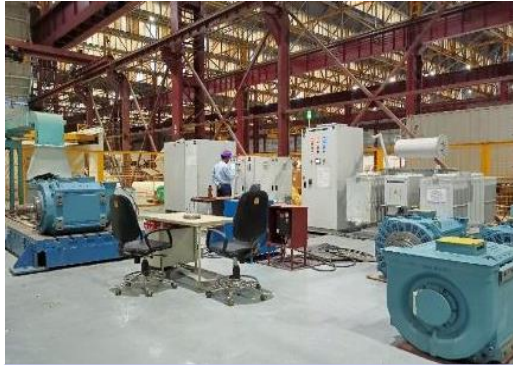
Traction Motor Testing facility
