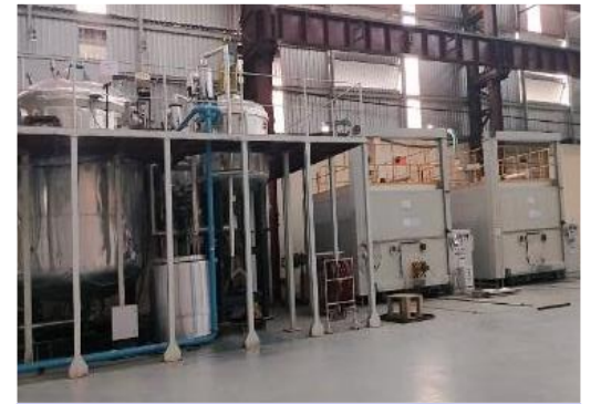
VPI Plant with Oven
