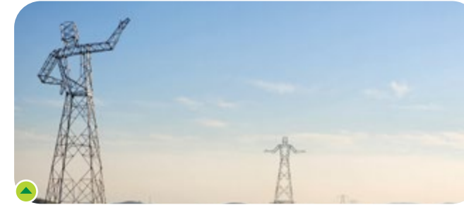
500 kV HVDC 200 km Transmission Line from Tajikistan Border to Afghanistan
