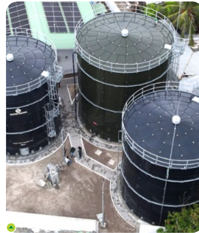
Construction of water and sewerage facilities including RTP and Admin buildings across 10 Maldivian islands.
