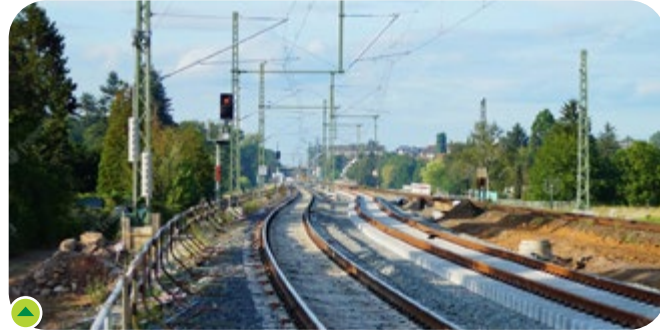
Antri Jhansi 3 rd Line Project is part of a larger 274 km Mathura-Jhansi line adding extra capacity to a key north-south corridor.
