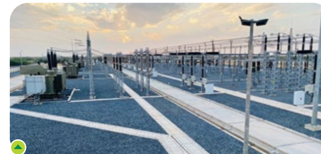
225/30 KV Substation in Senegal
