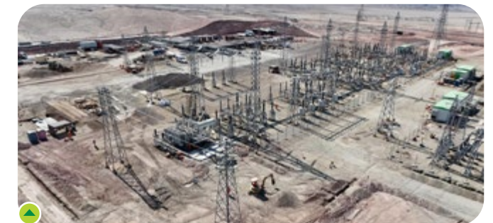
220/110 KV AIS Substation in Chile
