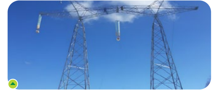
750 kV S-C 353 km Transmission Line in Ukraine
