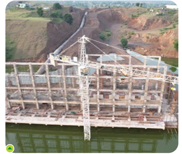
24 MLD Lahchura Water Supply Scheme in Uttar Pradesh
