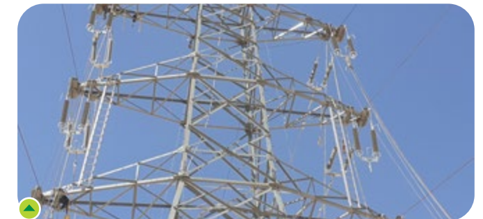
225 kV Double Circuit line in Mauritania
