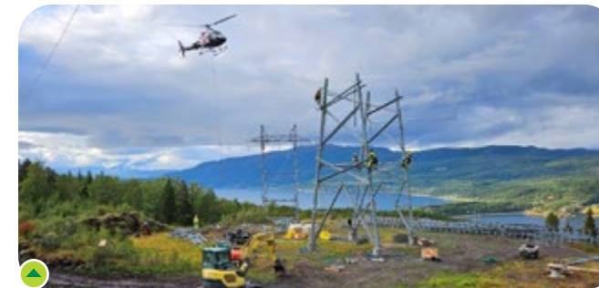
132kV S-C Transmission Line in Norway
