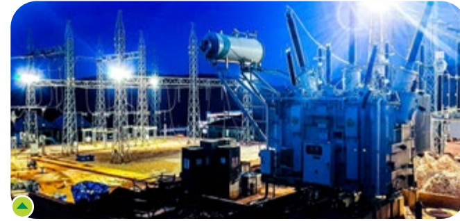
220-132 kV Substation in Burundi
