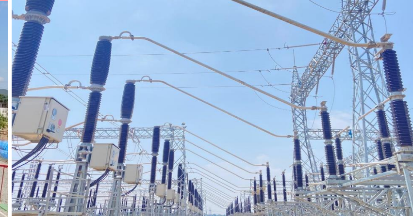
220kV, 132kV & 33kV substations for Intra-State Transmission, Madhya Pradesh
