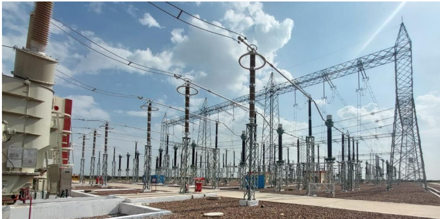
400kV, 600MW substation at Jaisalmer, Rajasthan
