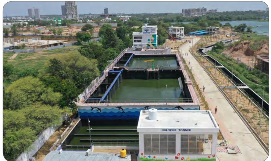
STP plant at Kokapet, Hyderabad (Hyderabad STPS Limited)
