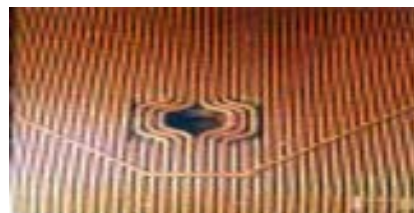
Water Wall Tubes
