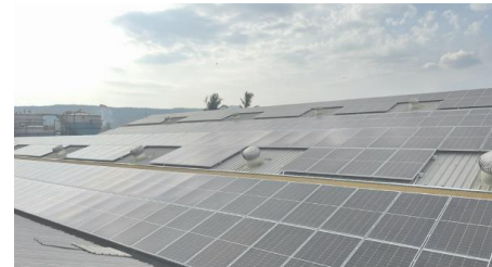
Rooftop Solar Panel
