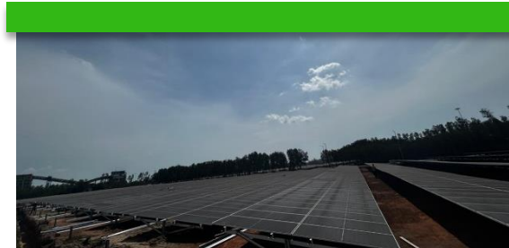
52.6 MWp Ground Mounted project at Simhapuri, Andhra Pradesh
