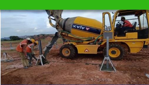
980 MWp Ground Mounted project at Pinnapuram, Andhra Pradesh
