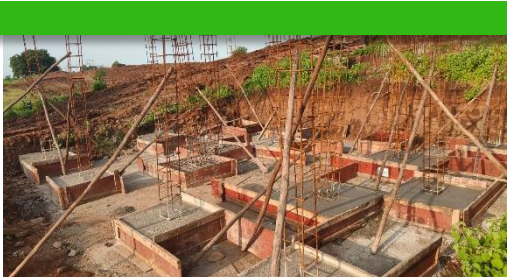
70 MWp Ground Mounted project at Jalna, Maharashtra
