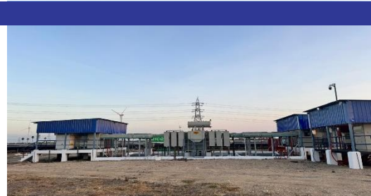
154 MWp Ground Mounted project at Thoothukudi, Tamil Nadu
