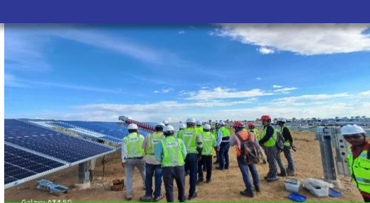
412.5 MWp Ground Mounted project at Bikaner, Rajasthan
