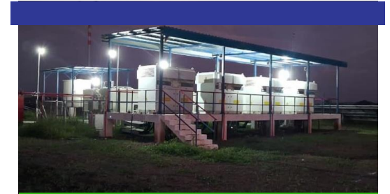
100 MWp Ground Mounted project at Jamnagar, Gujarat
