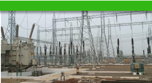
210 MWp Ground Mounted project at Khandwa
