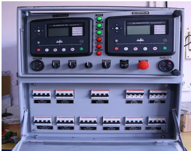
AMF Control Panels, Synchronizing Panels and Distribution Panels.
