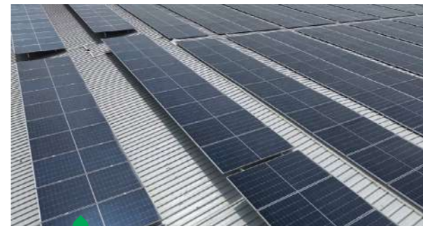
Solar Power At Rajkot Facility Capacity: 200 KW
