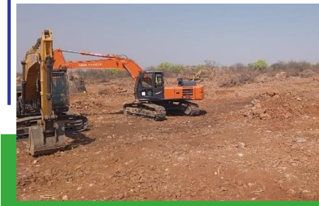
980 MWp at Kurnool, Andhra Pradesh
