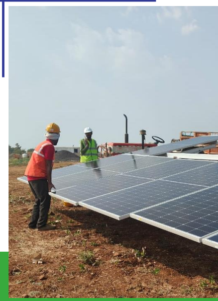
70MWp Ground Mounted project at Jalna
