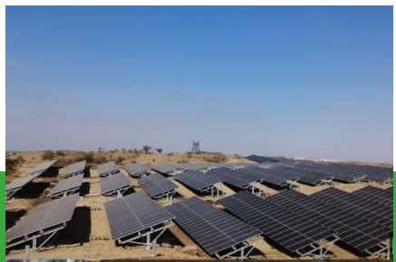
100 MWp at Jamnagar, Gujarat
