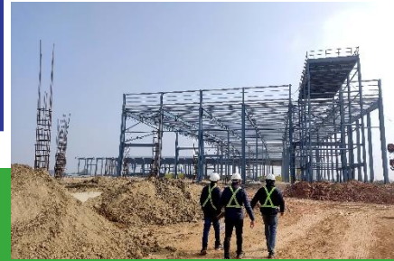
4.2 MWp Ground Mounted project at Rajasthan
