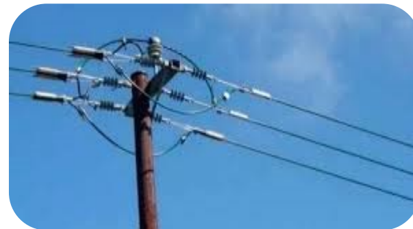
Covered conductor ( 20 km – 60 km from coast)
