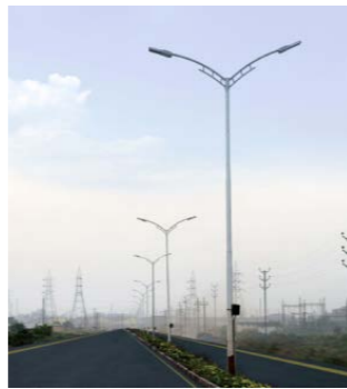
Lighting Poles and Masts
