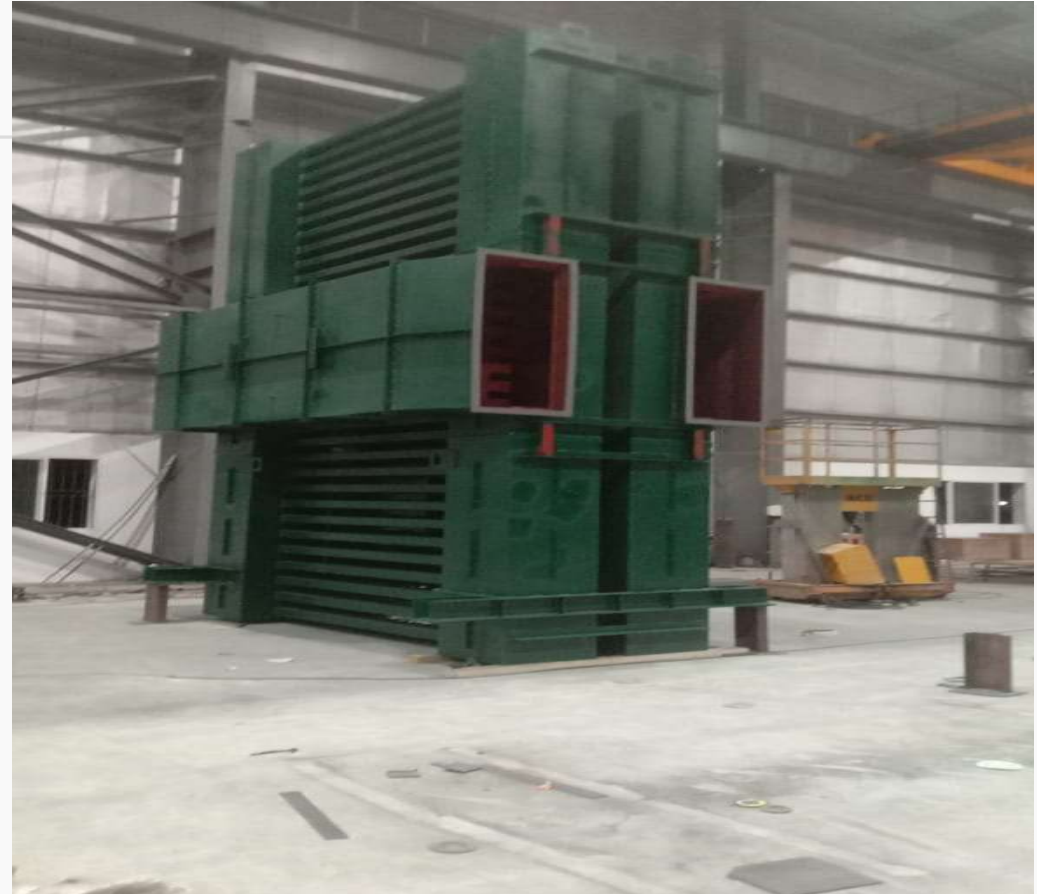
Biomass Pellet Structures for Pellet Plant
