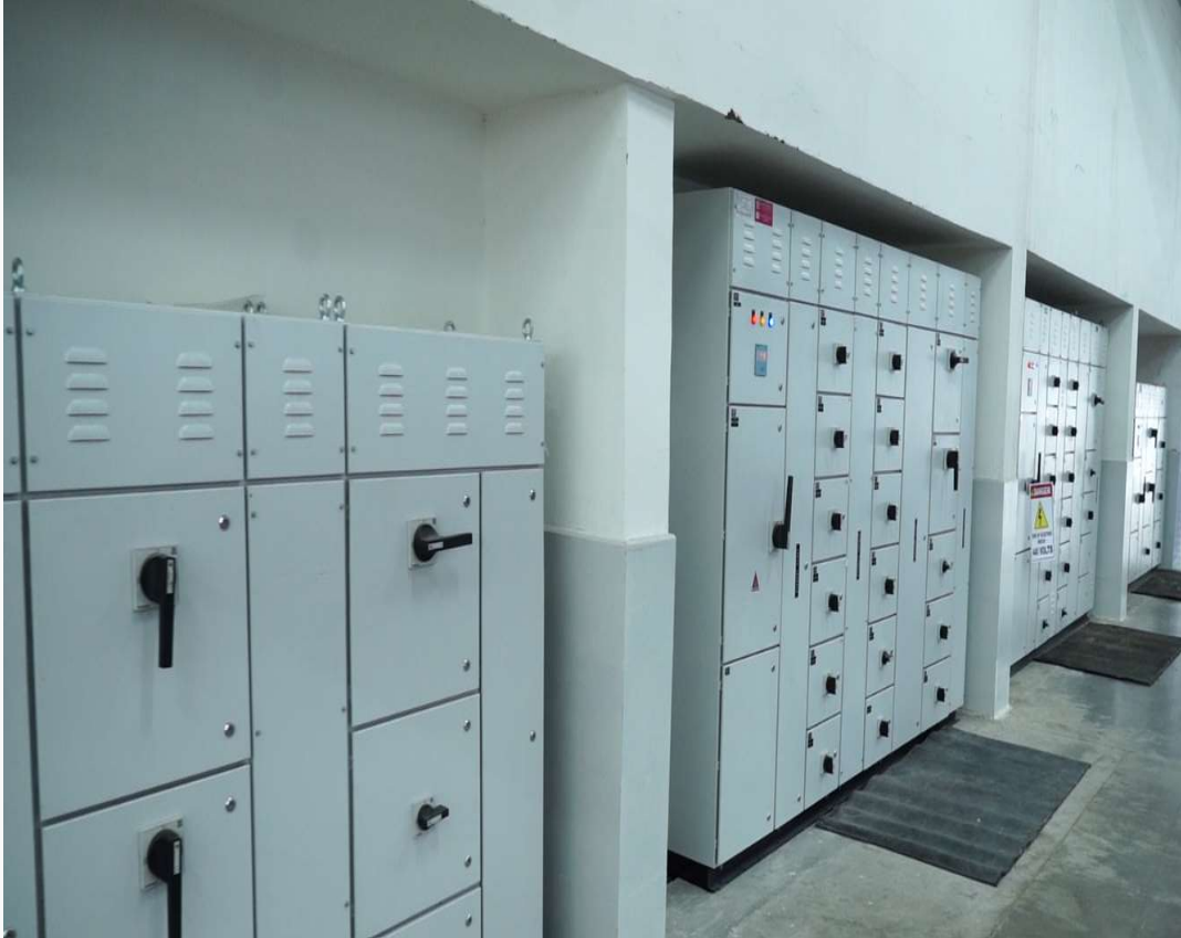
Electrical Panel Supplied for Spinning Mill – Bhagirathi Textile, Nagpur
