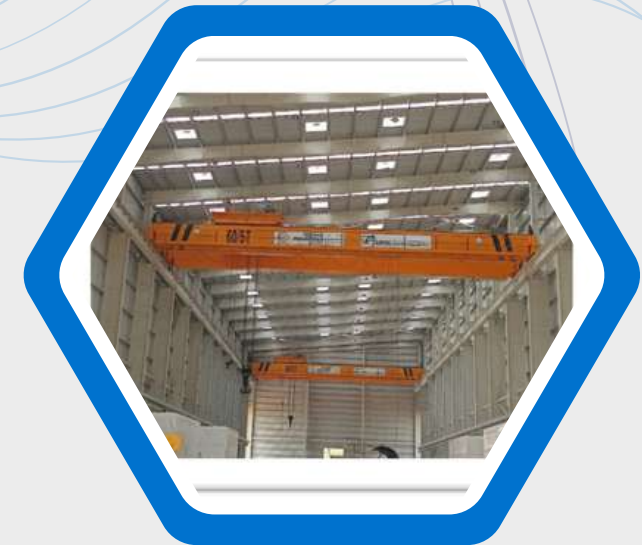
Electric Overhead Travelling Crane (EOT)
