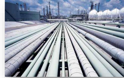
Anti Corrosive Material
