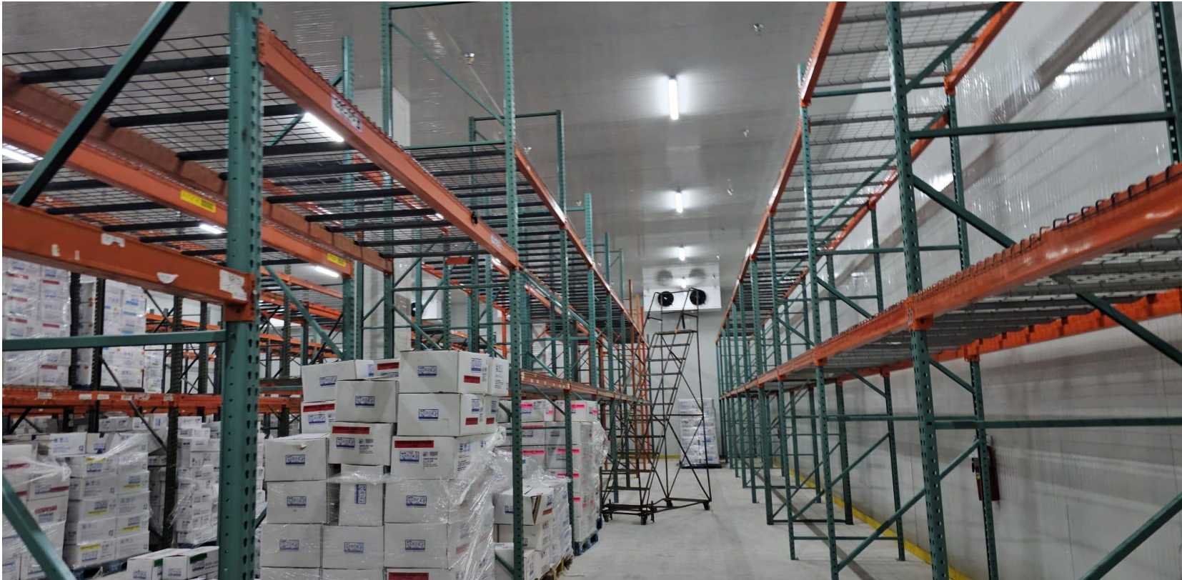
Cold storage facility in New Jersey, USA
