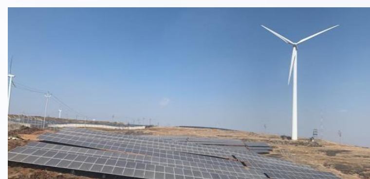
Solar Power Plant Ahmednagar, Maharashtra (5.2 MW)
