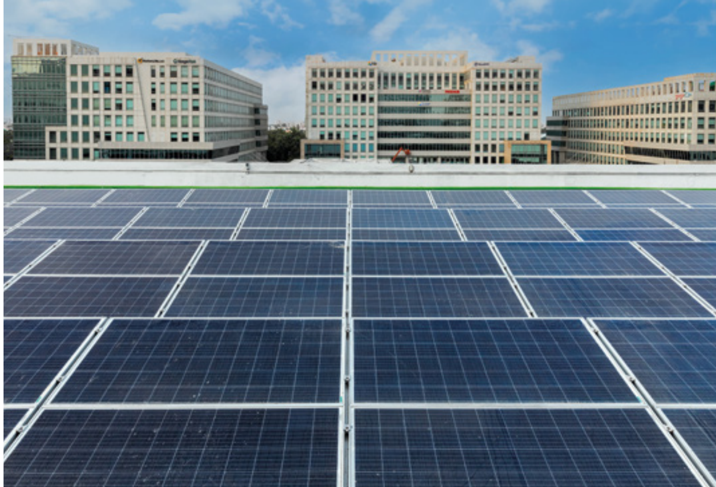
▲ Solar Panels installed at DLF Cyber City, Chennai
