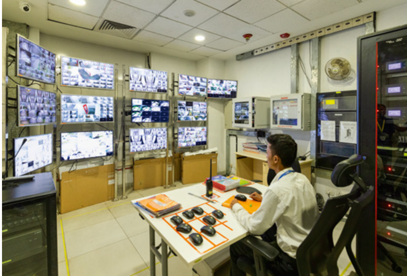
▲ CCTV Monitoring at Cyber City, Chennai
