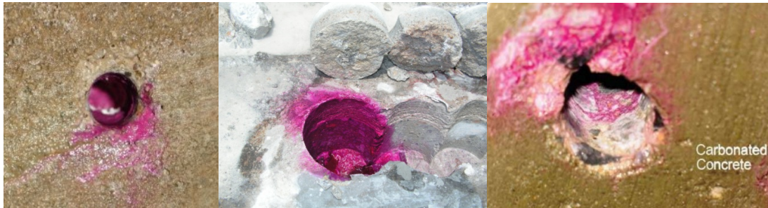
Fig.2.10: Images showing Carbonated concrete
