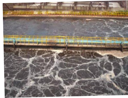
Diffused Aeration System
