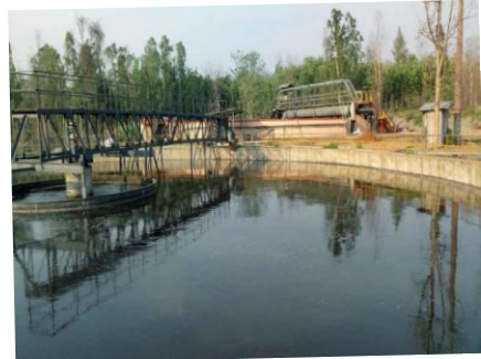
Secondary Clarifier - Pulp
