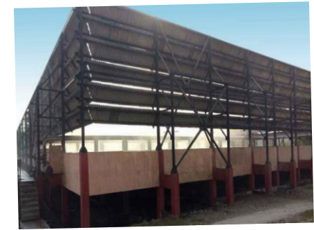
Mist Cooling System
