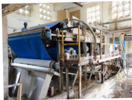
Sludge Handling - Paper
