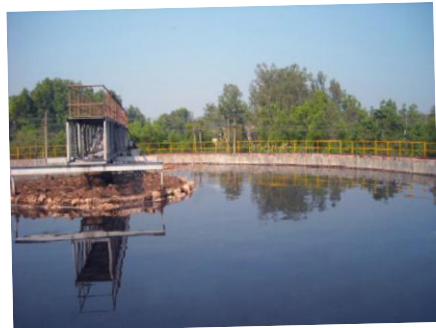
Primary Clarifier - Paper
