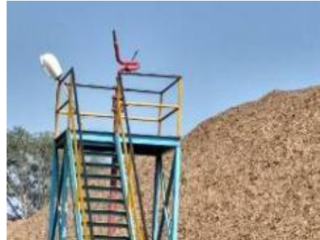
Fire Hydrant Point near chipper
