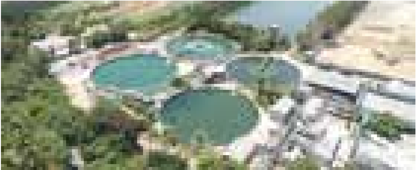
Waste water treatment plant
