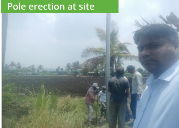
LT Line with Stud pole
