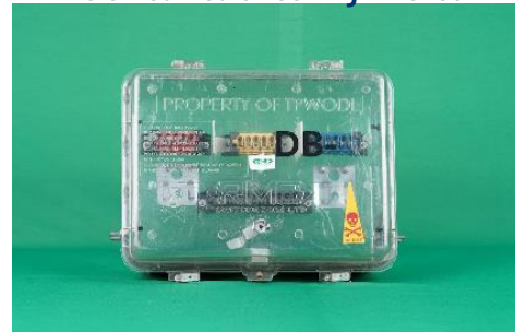
Pole Mounted Street Light Boxes
