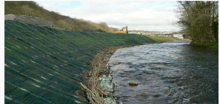
River Bank protection/erosion control measures on the left bank of river Subansiri adjacent to village Gerki - 2 (RD 29 KM to - 30 KM)
