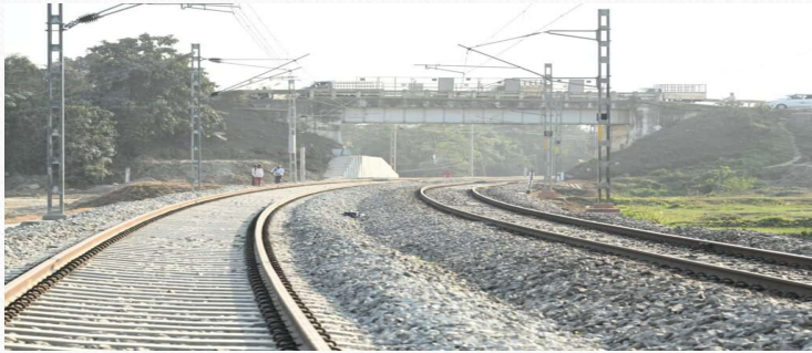
Construction of sub-structure and super-structure on pile foundation of major bridges in connection with double line work of New Bongagaon-Agthori doubling project.
