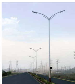
Lighting Poles and Masts
