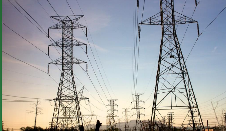
Power and Transmission
