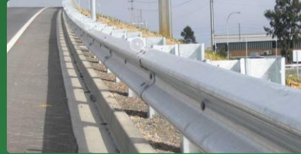
Metal Beam Crash Barrier
