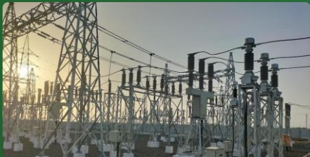
Sub-Station Equipment Structure
