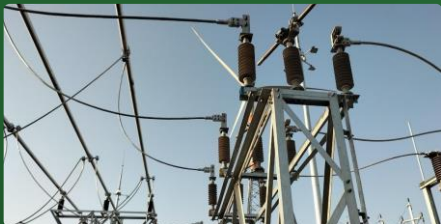
Isolator (HV Disconnectors)
