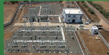
Pooling Sub-Station Development
