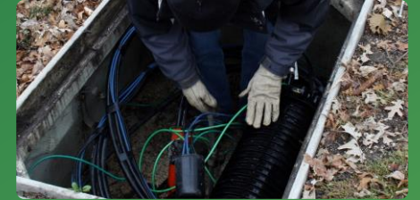
Optical Fiber Fault Rectification
