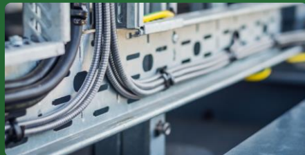
Cable Tray & Earthing Material
