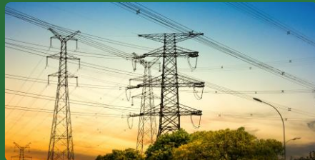
Transmission Line Tower
