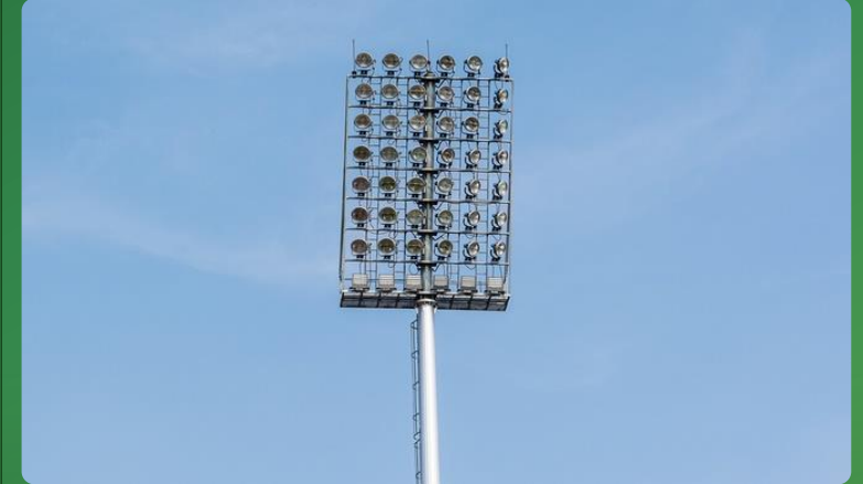
High Mast Poles & Lighting Poles
