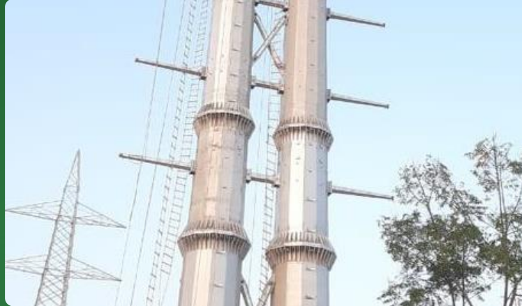
Transmission line Monopoles
