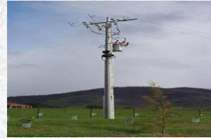
Power Distribution Poles
