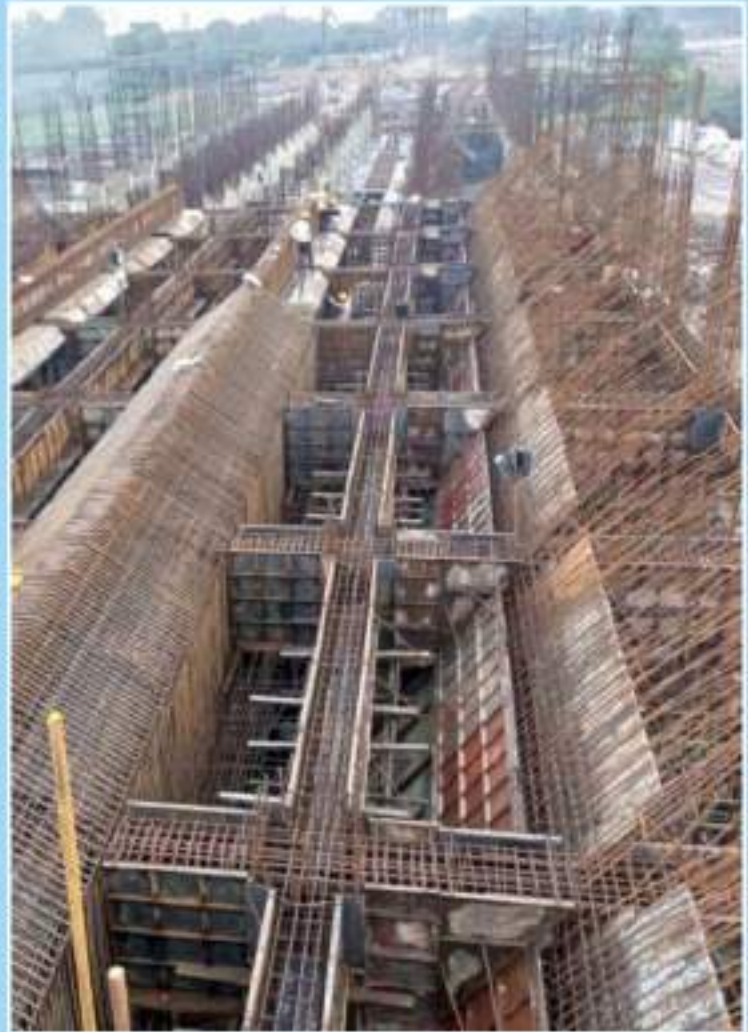
Construction of 20000 tonne capacity over ground coal storage bunker for 9.50 MTPA NCL BINA KAKRI Project is under progress
