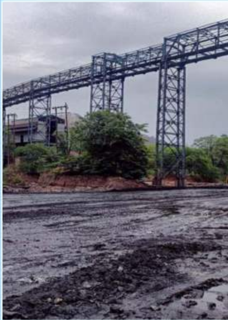
Central Conveyor (CC-4): Technological Structures & Arrangement of Belt Laying in Progress at Nigahi 10.00 MTPA OCP CHP Project in Madhya Pradesh
