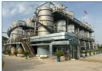
2 MLD Leachate Treatment Plant, Hyderabad, TS
