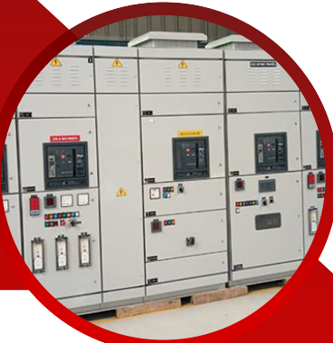
Control Panels & Distribution Panels
