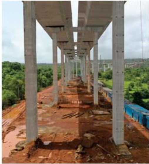
The elevated corridor consists of numerous piers that reach height of up to 40 meters.
