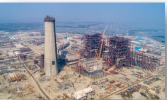
2X660 MW at Rampal, Maitree, Bangladesh-BIFPCL
