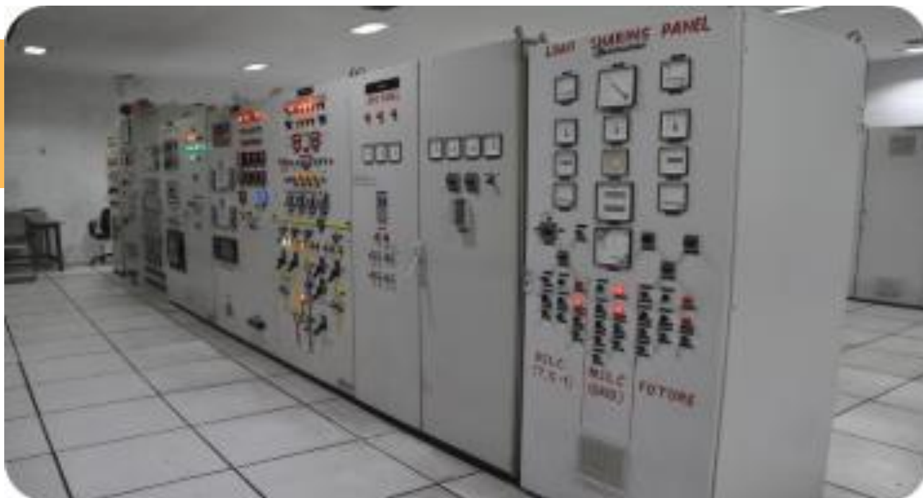
Cogeneration control panel
