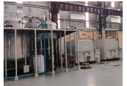
VPI Plant with Oven
