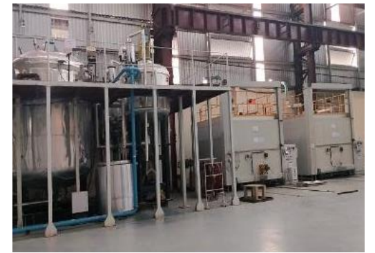
VPI Plant with Oven
