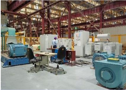
Traction Motor Testing facility
