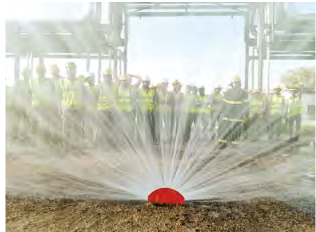
Sprinkler demonstration being given for Fire Safety Drill at BCML
