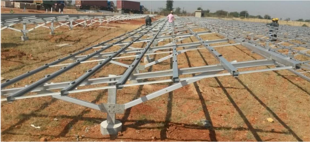
Module Mounting Structure
