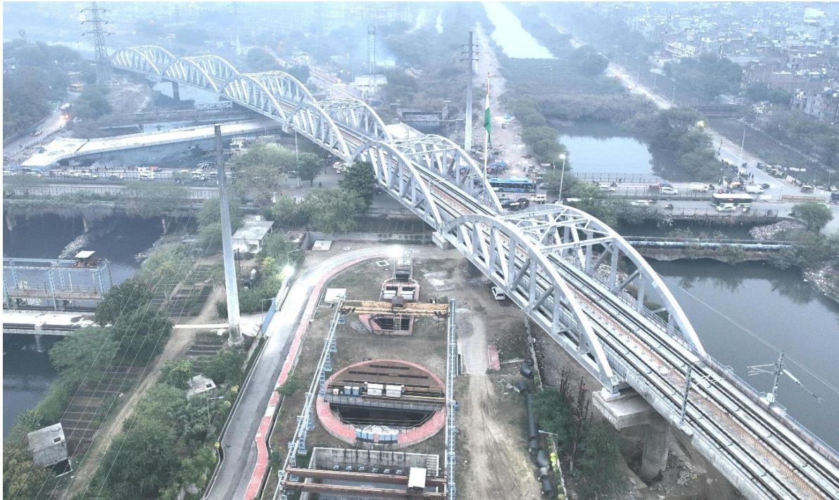
The six special bow-string steel spans on the Delhi-Meerut Namo Bharat Corridor Package-6
