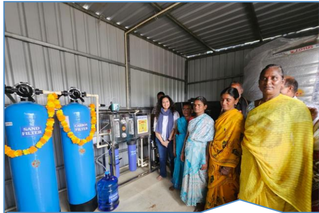
Access to safe drinking water with 9 new RO plants taking total to 63.
