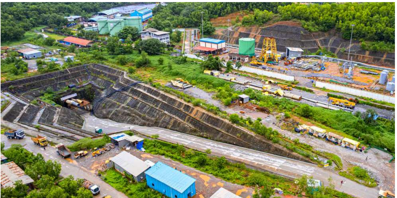
LPG cavern at Mangalore, Karnataka
