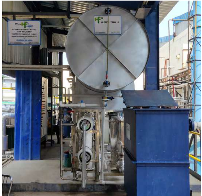
Zero liquid discharge process at UFlex's chemicals plant in Noida, Delhi NCR, India
