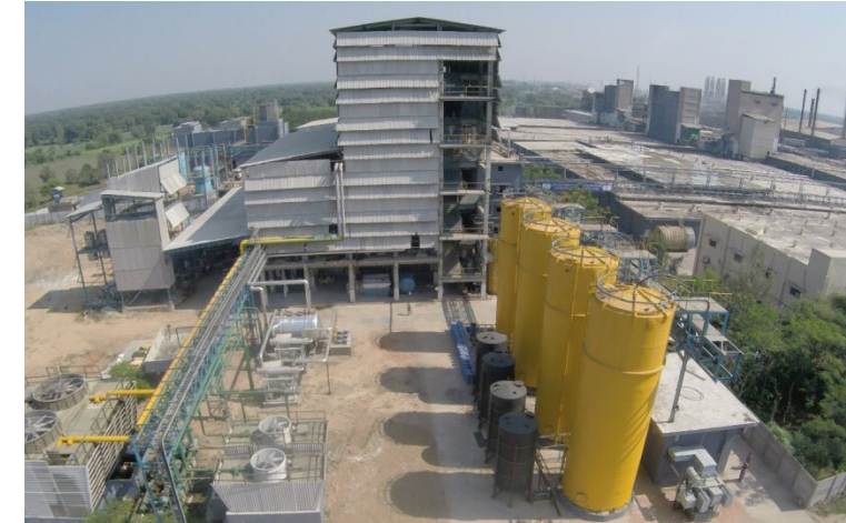
Multiple Effect Evaporator Plant (MEEP)
