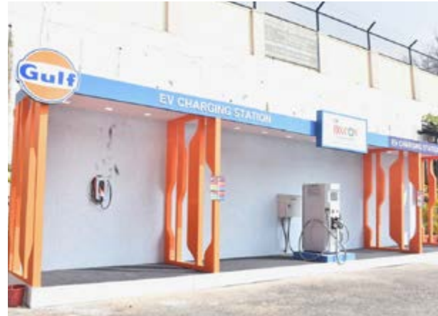
EV Charging facility powered by Gulf Oil
