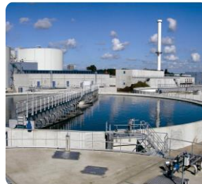
Water & Waste water management
