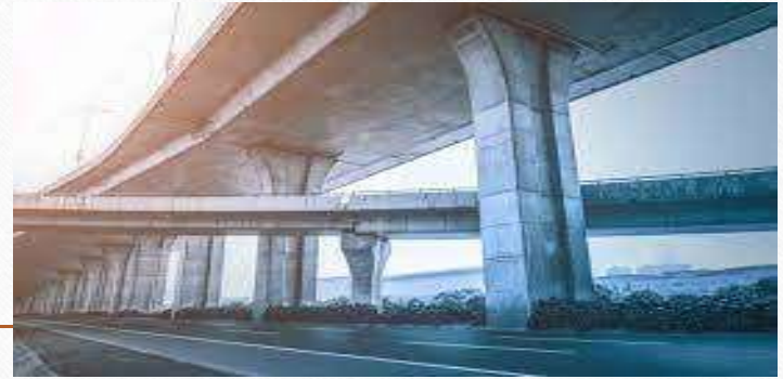
Maintenance of 3 lane Brahmaputra Bridge including their expansion joints & bearing, providing all necessary signboard, road furniture etc..
