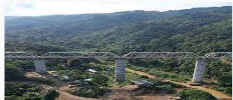
Construction of foundation and sub structure over pile foundation for Tall Bridge of new BG Railway line from Bairabi to Sairang (Mizoram).
